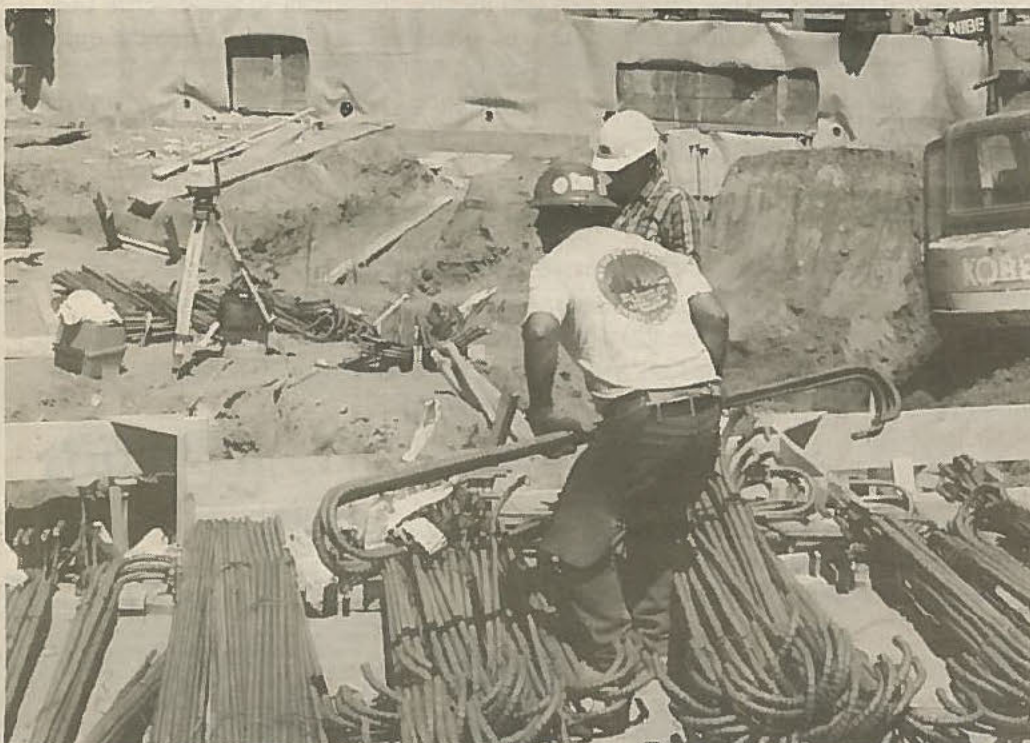
At 20% complete, the metal reinforcements are being put in place for the concrete foundation and in preparation to start erecting the steel structure.
